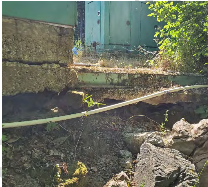
Photo 2: Subsidence under Hotel Well surface seal
