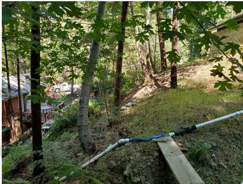
Photo 13: Failing Luther Tank in relation to house located downhill.
