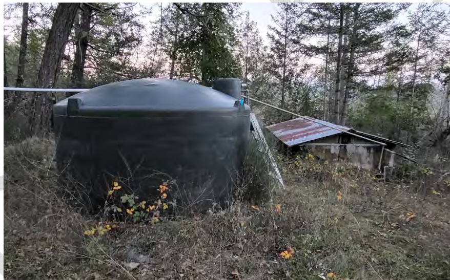
Photo 5: Transmission tanks upstream of the Buckeye Tank
